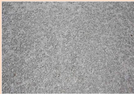
Affected by Chemical Spillage
