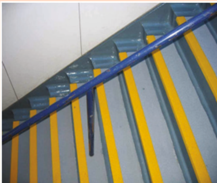
Safety Staircase with Nosing
